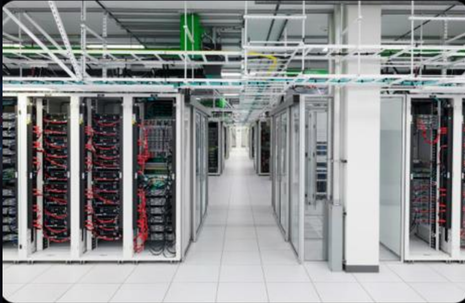
Traditional Cloud Data Centre
