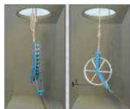
Sheaves and quadrant block in manhole
