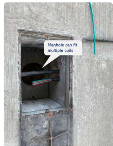
Manhole size is critical
