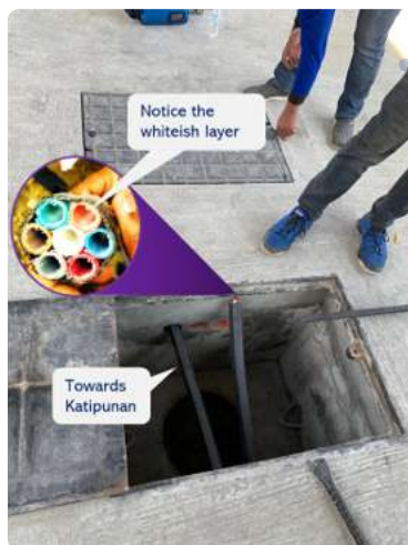
7 way 16/13 mm bundled duct
