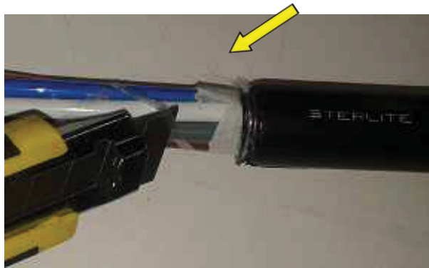
Figure 16- Removal of the binding tape which bundles tubes in cable core using blade knife
