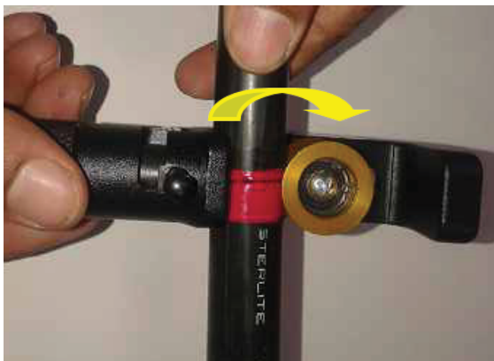
Figure 3- Cable sheath being ring cut at the 15 cm window near the center of mid-span access window
