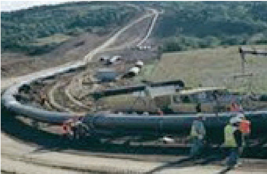
Sterlite fiber optic cables deployed in India's longest natural gas pipeline
